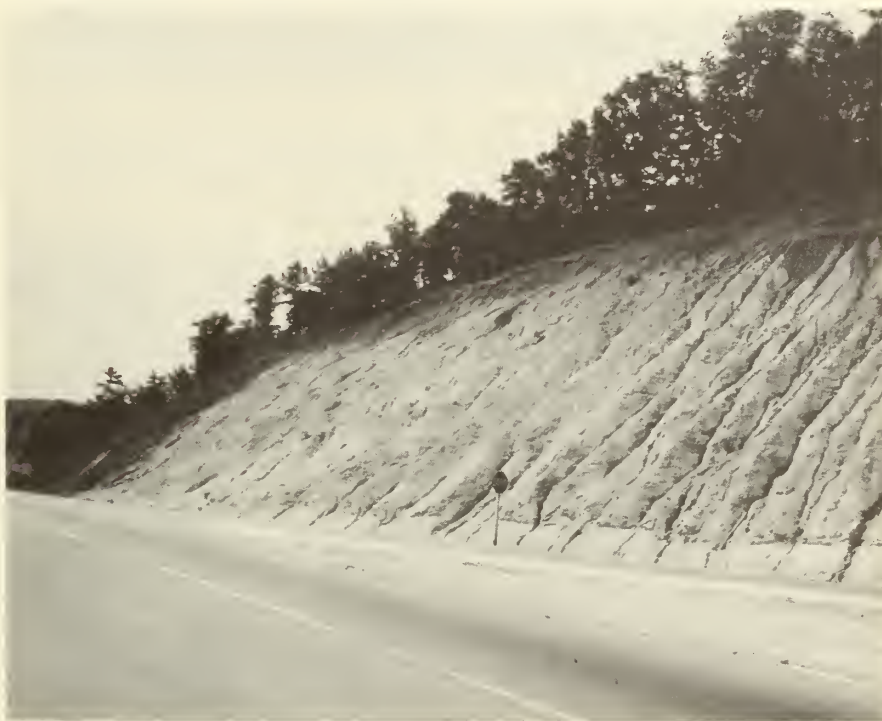
Figure 1.--A common sight on unprotected road cuts throughout the United States, particularly in the Southeast.
